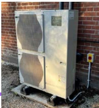
Newnham College Air Source Heat Pump
